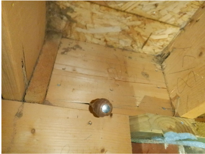
Photograph Number 3 - View of termite damaged block located at end of the joist that needs repair. Remove, probe framing behind it and repair as needed.
