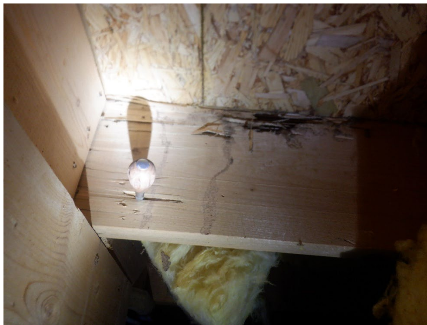
Photograph Number 2 - View of termite damaged end of floor joist where a full length "sister" joist should be installed as a repair.
