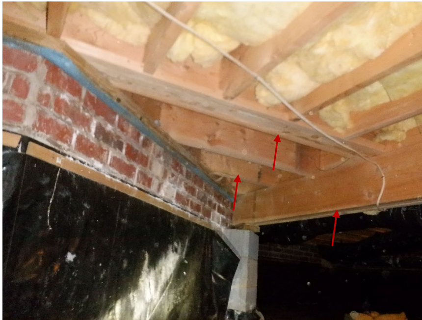
Photograph Number 1 - View of area of floor system where minor termite damage was observed.
